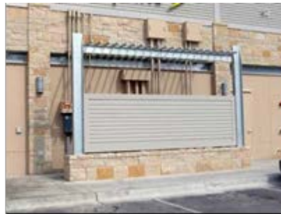
Utility equipment in more visible location screened by wing wall
